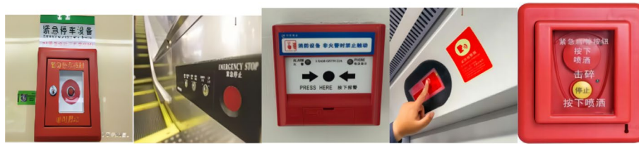
Fig. 1 Subway Emergency button a Emergency stop b Emergency stop c fire alarm d vehicle emergency intercom e gas fire extinguishing
